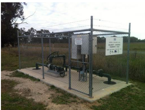
Salinity control pump site CG23 north of Byrneside
