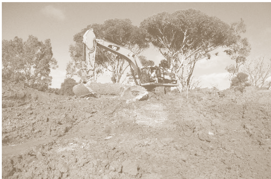
Replacing 5 subways along the Waranga Western Channel between the 74km and 85km regulators.
