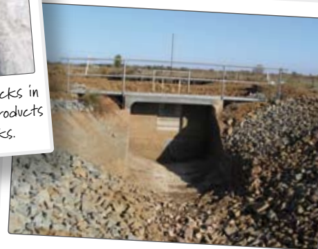
Beaching Reinstating eroded beaching. Poor quality material is removed and replaced with selected clay, then covered with geofabric and rock beaching.
