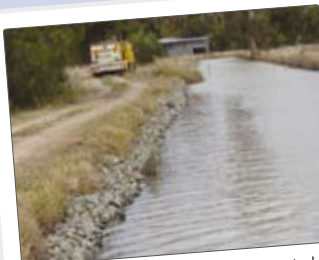
The inside of the channel bank batters is shielded from erosion by applying a thin protective layer of rock.
