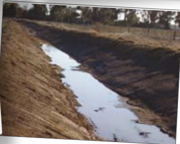
Eroded bank material from the bed of the channel is reinstated onto the inside of the channel bank batter, creating a stable slope which slows the rate of deterioration.
