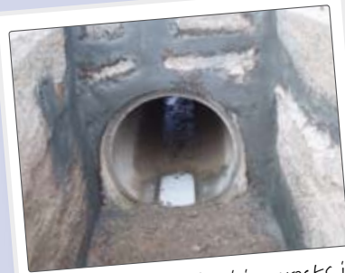
Structural Repairs: Repairing cracks in concrete structures with epoxy products adds stability and deters leaks.
